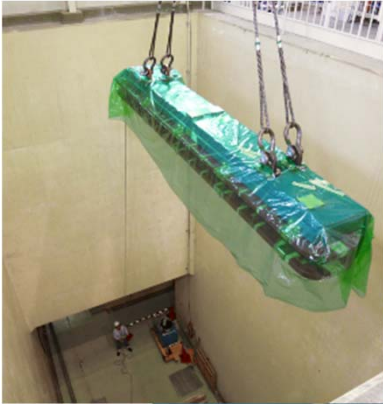
Installation of 100 new long LER bending magnets
