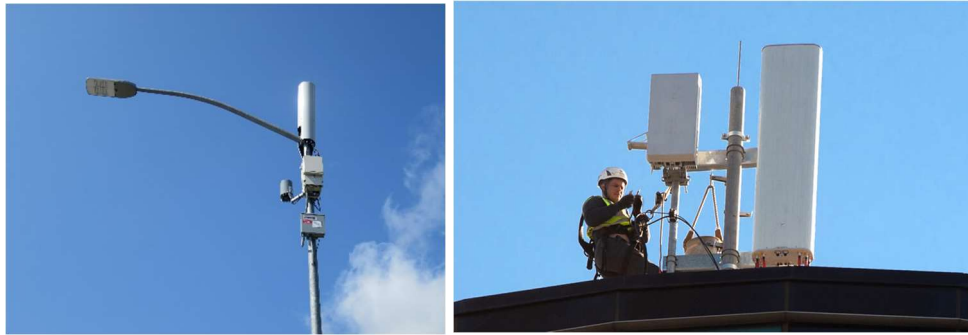
Fig.3: Examples of base station antenna systems of new generation. During the transition period both old and new systems will be operating alongside each other.
